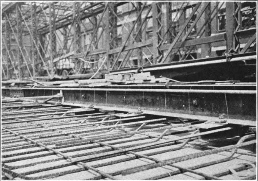
Figure 6. Harrison Street Viaduct, showing old viaduct and the relation of the tracks to the concrete reinforcement of the new viaduct.
